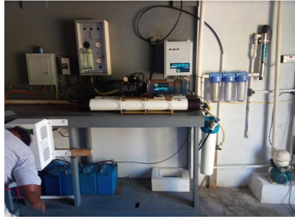
Figure:3 RO Unit Installment Enewetak Atoll
